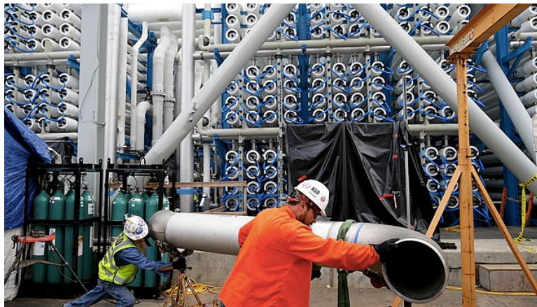
Figure 39. Carlsbad, California Reverse Osmosis Desalination Project's 10-mile water pipeline uses 2,000 pressure vessels and is the largest desalination plant in the Western Hemisphere.
