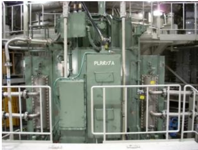
Figure 11. BWR primary coolant recirculation pump. Source: Tepco.
