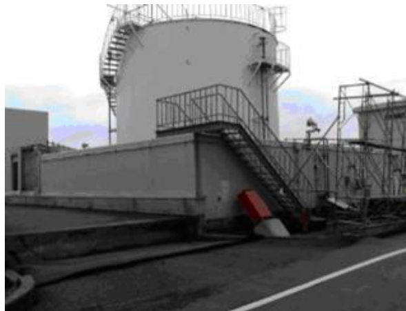
Figure 33. Earthquake-caused ground subsistence around light oil storage tank of 30,000-40,000 gallons capacity, 1979. Source: Tepco.
