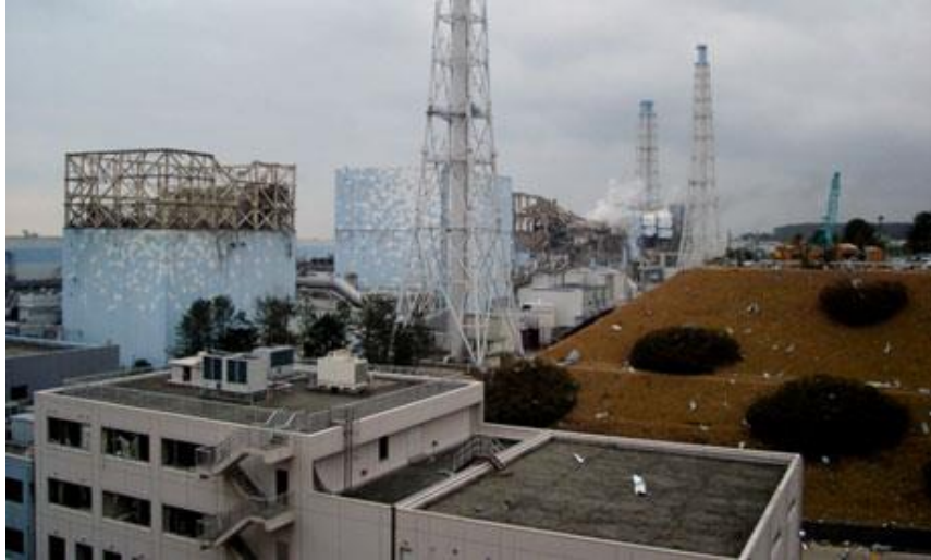
Figure 52. Damage to the upper structure of the Fukushima Daiichi unit 1, and undamaged structure of unit 2. Source: Tepco.
