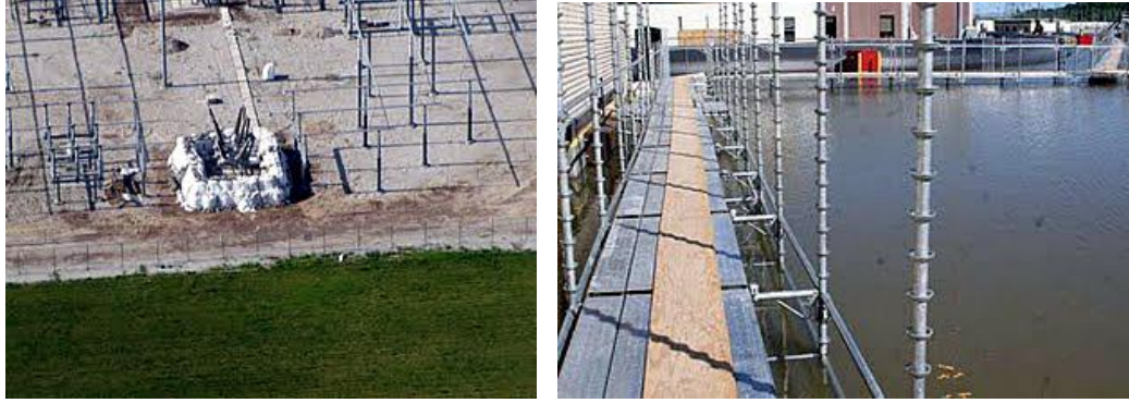
Figure 89. Circuit breaker 345 kV at transformer substation protected with sandbags and walking bridges around buildings were implemented against flooding at Fort Calhoun, Nebraska, June 13, 2011. Source: OPPD.
