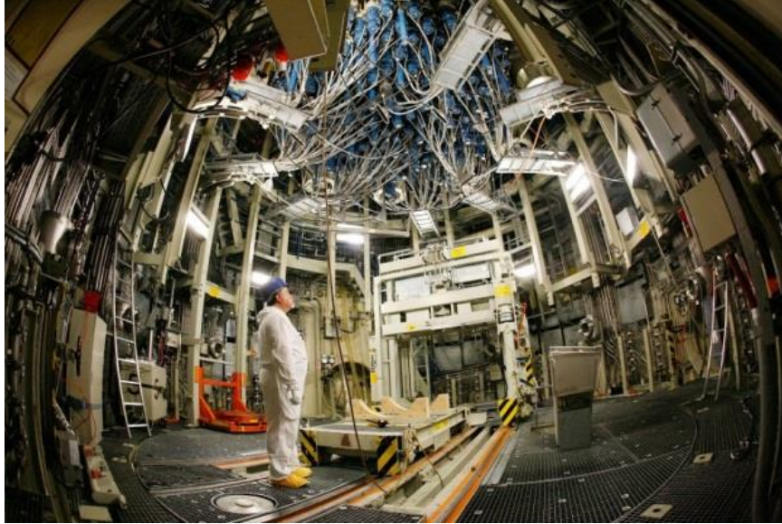
Figure 90. Control rod drives at the bottom of the Krümmel BWR reactor near Hamburg, Germany that went into operation in 1984.
