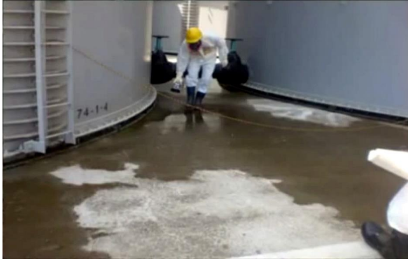
Figure 92. Leaking water storage tanks.
