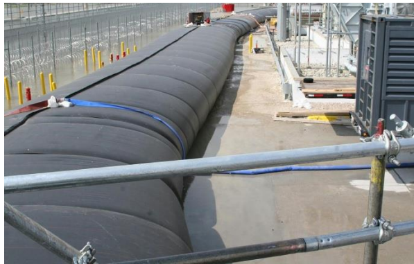
Figure 87. Fort Calhoun station, Blaine, Nebraska, 19 miles north of Omaha on the Missouri River is protected against flooding by a 2,000-ft long Aqua Dam berm from releases from the Gavins Point Dam, June 10, 2011. The berm raises the protection 6 ft above the 1,004 ft river level to the 1,010 ft Mean Sea Level, MSL. Source: OPPD.
