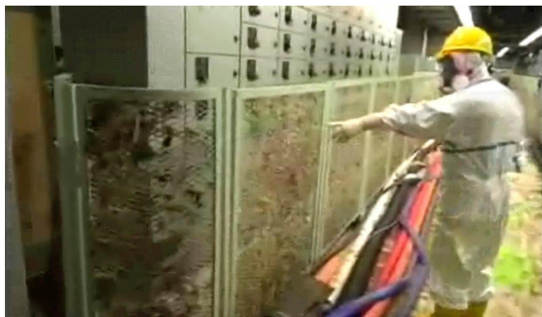
Figure 47. Tsunami water flooding of electrical switching components in basement of unit 1, May 6, 2011. Source: Tepco.
