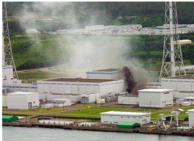
Figure 69. Burning electrical transformer resulting from the coupled earthquake and tsunami event, March 11, 2011. Source: Japan Coast Guard.
