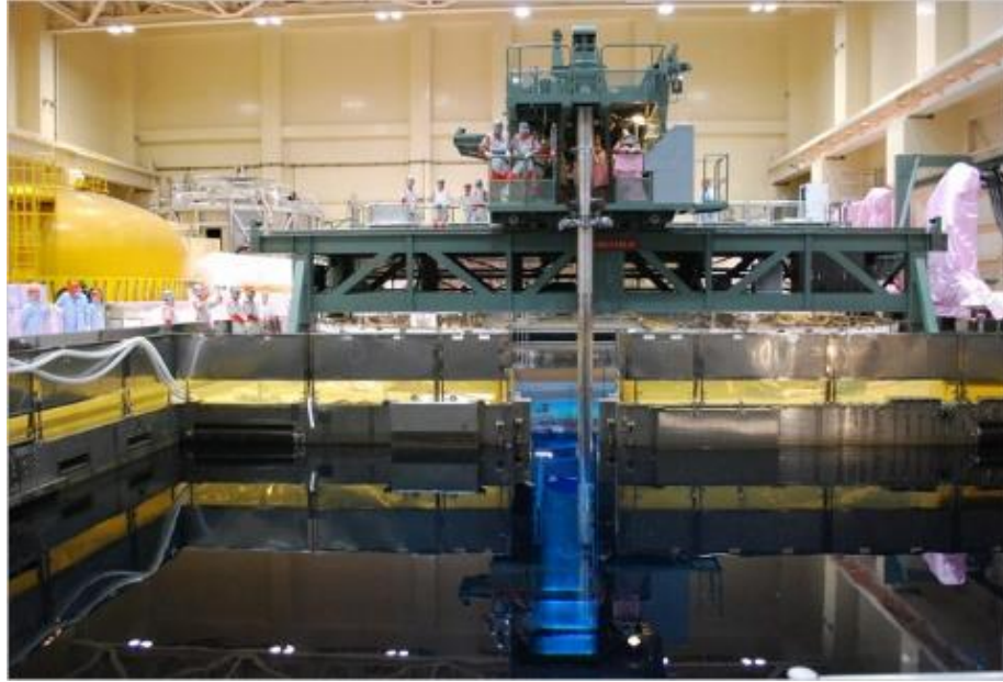
Figure 51. Refueling operation into fuel storage pool. Yellow object is the removed core dome.
