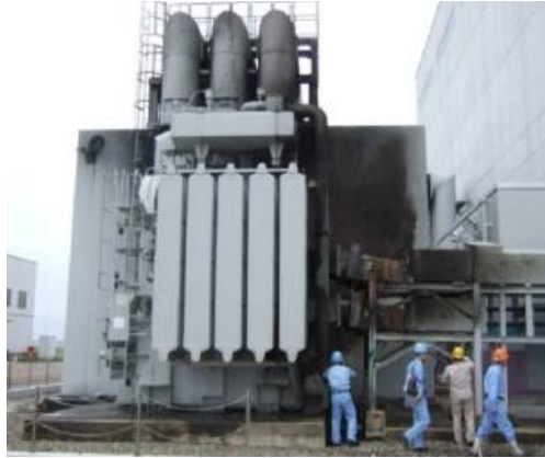
Figure 37. Transformer fire caused by 1979 earthquake. Notice the location of the transformer outside the plant enclosure and its vulnerability to water-flooding from the tsunami event. Source: Tepco.
