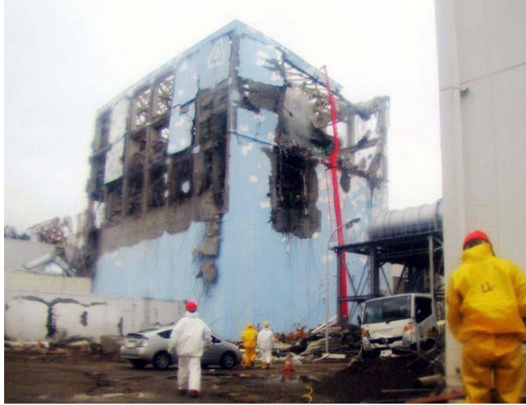
Figure 84. Damage below the fuel storage pool in unit 4 as seen from the ground on March 22, 2011. Water being pumped into the damaged spent fuel pool using a boom. Source: Tepco.
