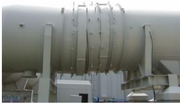
Figure 34. Earthquake-caused displacement of connecting duct to the main ventilation stack, 1979. Source: Tepco.
