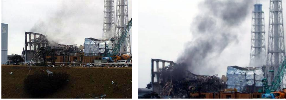
Figure 54. Fukushima Daiichi Unit 3. Steam emission on March 21, 2011 evolved into black smoke. A possible hydrogen or steam explosion tore out the upper part of the containment building structure. The blow-out-panels are missing, with remaining steel and concrete beams. The reactor containment vessel is reported to remain intact, even though the nuclear fuel storage pool and the reactor refueling deck would be exposed to the elements. Steam and dark smoke emanating from possible burning of the \text{UO}_2 fuel, concrete rubble, or boron carbide \text{B}_4\text{C} embedded in the Al of the Boral shielding material if it is used in the fuel storage pool as spacer between the fuel assemblies. Source: Tokyo Electric Power Company.
