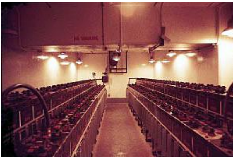
Figure 33. Emergency Battery Banks for backup power.
