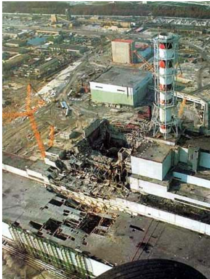
Figure 1. Damaged unit 4 of the Chernobyl plant, before being enclosed in a concrete silo.
