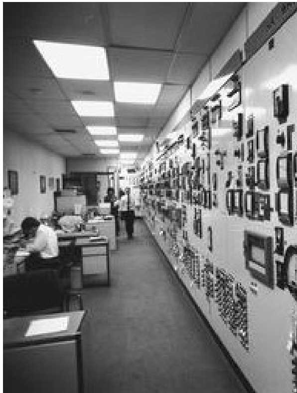
Figure 21. Reprocessing canyon F control room.
