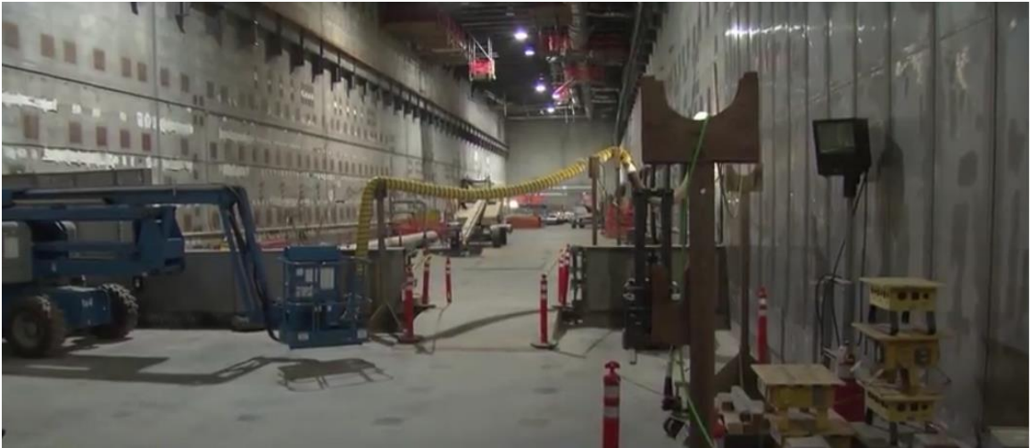
Figure 38. Interior of Purex Pu reprocessing plant canyon, Washington, USA.
