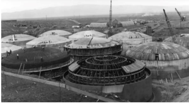
Figure 45. Double-walled high level waste tank farm at the Hanford reservation site, Washington, USA.
