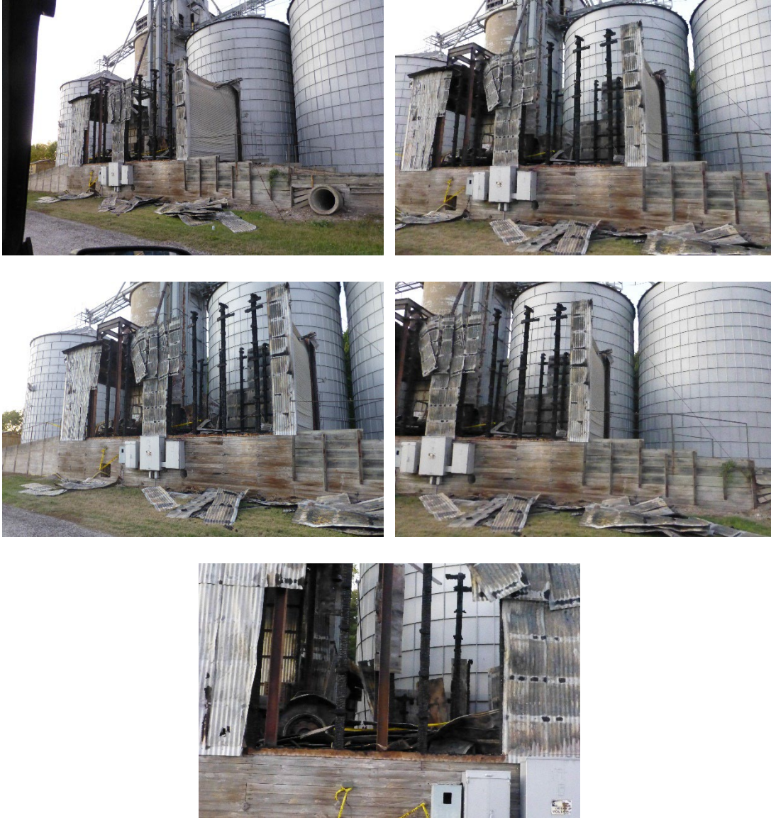
Figure 118. Suspected dust explosion and fire aftermath, Broadlands Grain Elevator, Illinois, summer 2013. Photos: Barbara Ragheb.
