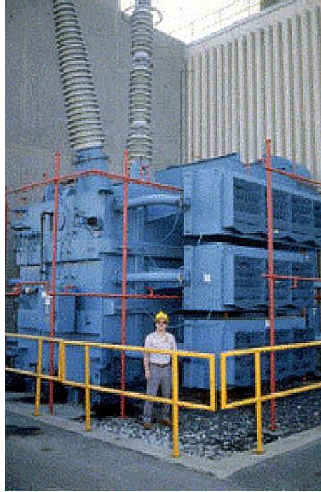
Figure 17. Damage to electrical transformers from the March 13, 1989 solar event.
