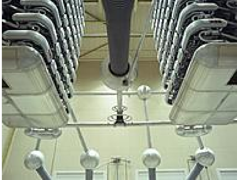
Fig. 2: Huizhou valve hall, Three Gorges Guangdong Transmission China.
