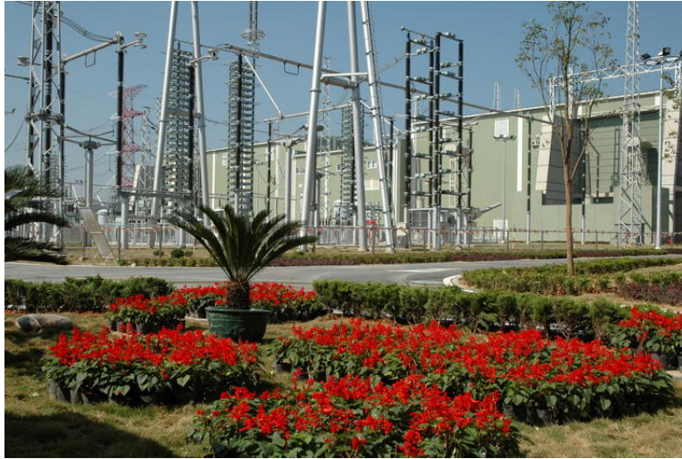
Fig. 1: Yidu station at the 3,000 MW Three Gorges project Shanghai China.
