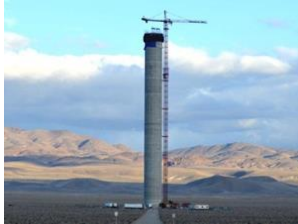
Figure 50. Solar reserve Crescent Dunes 110 MW, Tonopah, Nevada solar plant uses 10,000 billboard-size mirrors and thermal energy storage in a molten salt.
