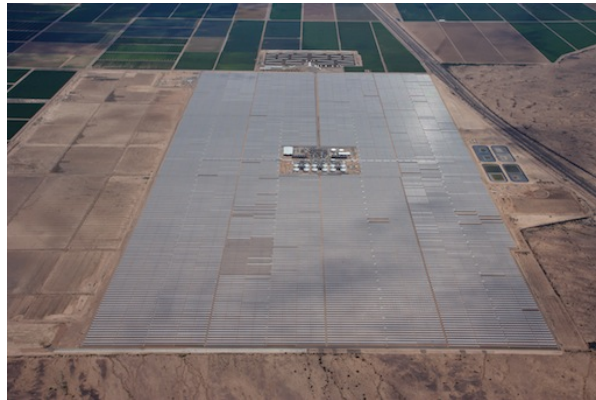
Figure 34. Solana 280 MWe power plant, Arizona, USA. Source: Abengoa Solar.
