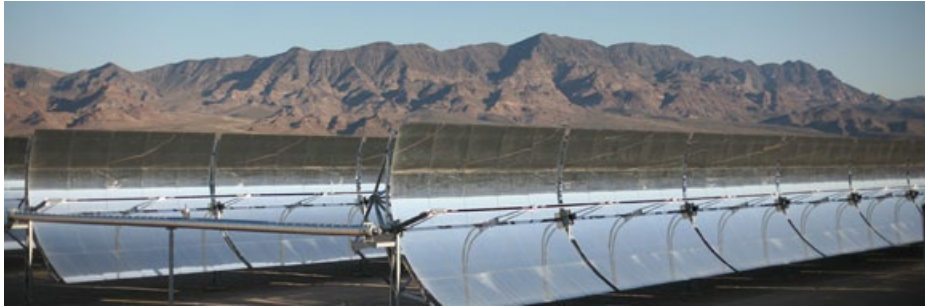
Figure 32. Nevada Solar 1 power plant. Source: Acciona.
