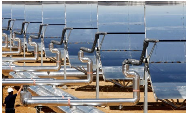
Figure 33. La Florida solar thermal power plant, Alvarado, Badajoz Spain. Photo: Reuters.
