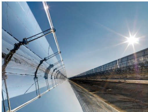
Figure 35. Parabolic collectors at the Solana Plant, Arizona, USA. Source: Abengoa Solar.
