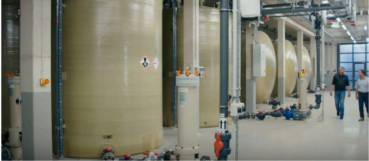
Figure 18. Large scale Redox flow batteries can store energy from consumer-owned DC current-producing wind turbines over long time periods without being connected to the grid.
