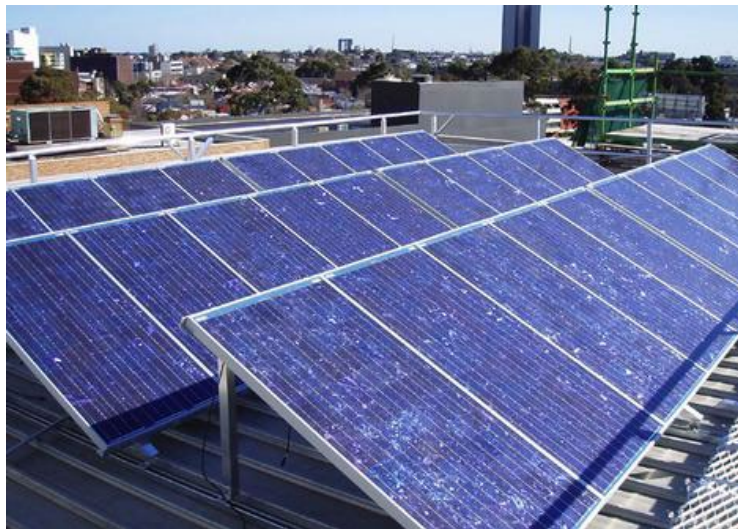
Figure 19. Photo Voltaic (PV) Solar collectors atop a building.
