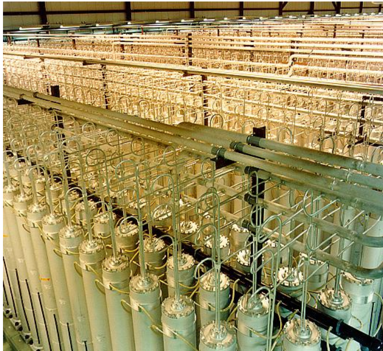
Figure 23. Urenco U 235 enrichment gas centrifuges cascade.
