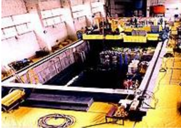
Figure 6. Fuel storage pool of Yongbyon-1, 5 MWth research reactor in the DPRK. AP Photograph.
